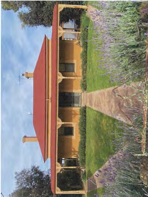
411 Light Pass Road 11 posts to be replaced on the front & left & right-hand side of building.
