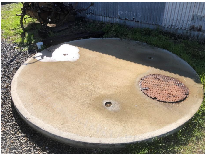
Figure 7 Wastewater holding tank.
