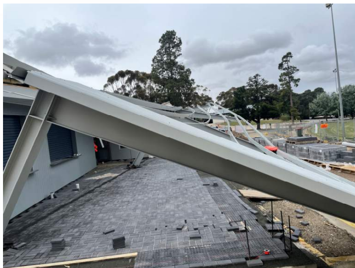
Photograph 3: Roof purlins have typically failed throughout due to the primary structure failing.
