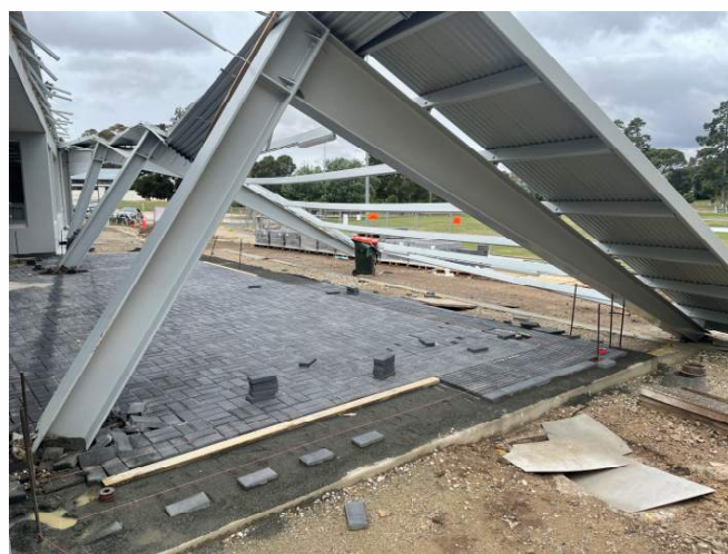
Photograph 2: The first three column/rafters from the most Southern end have collapsed. The four most Northern columns/rafters remain standing.
