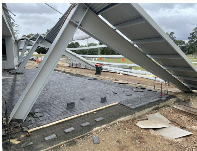
Photograph 4: The primary columns (310UC118) and tapered rafters (610UB101) do not appear to have failed.
