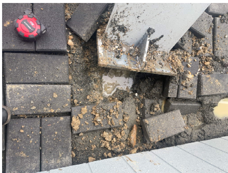
Photograph 8: The column base plate and gussets do not appear to have yielded. No evidence of waterproofing/protection to the column/base plate against corrosion.
