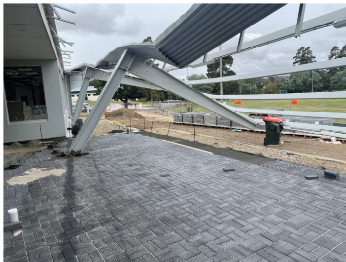
Photograph 5: The connection of the cantilevered rafter to column does not appear to have failed.
