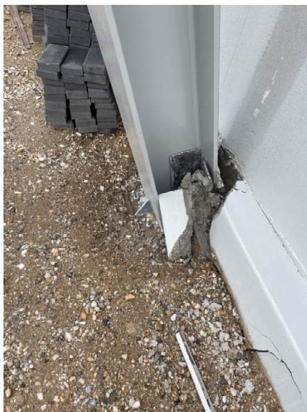
Photograph 9: The steel framed cantilevered structure located three in from the Southern end appeared to have an alternate base plate/bolt configuration than that of its adjacent columns that failed. Concrete failure to hob/footing upstand.
