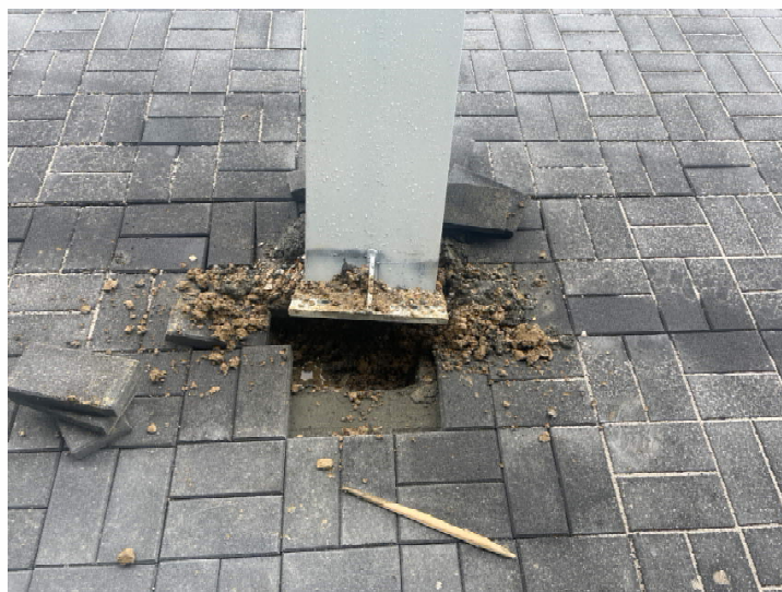
Photograph 6: The hold-down bolts have failed in tension.
