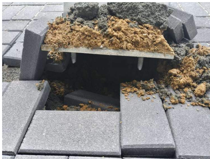
Photograph 7: The hold-down bolts have failed in tension.
