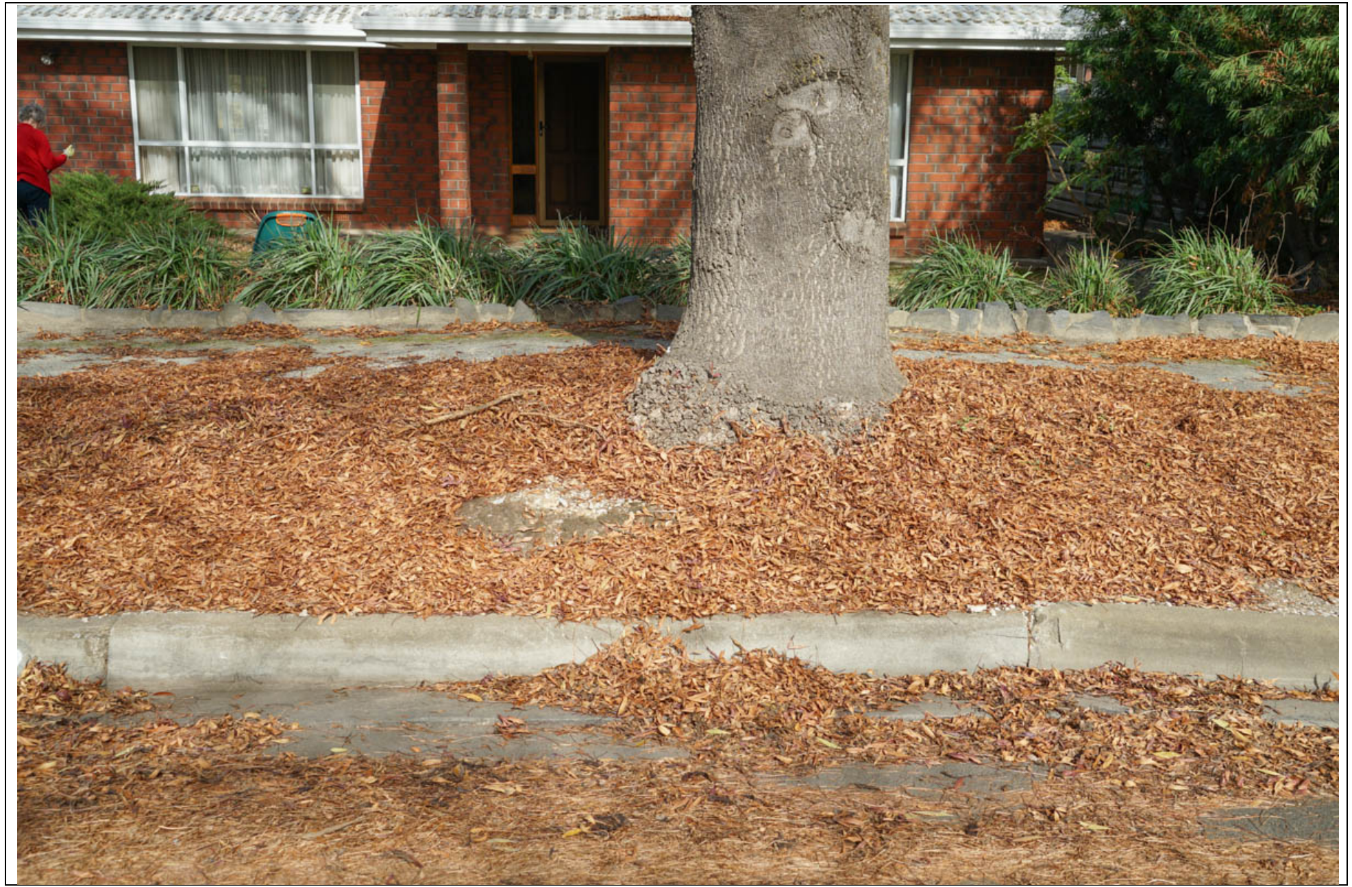
Photograph showing the major kerb and water table displacement adjacent to the stem of the tree.
