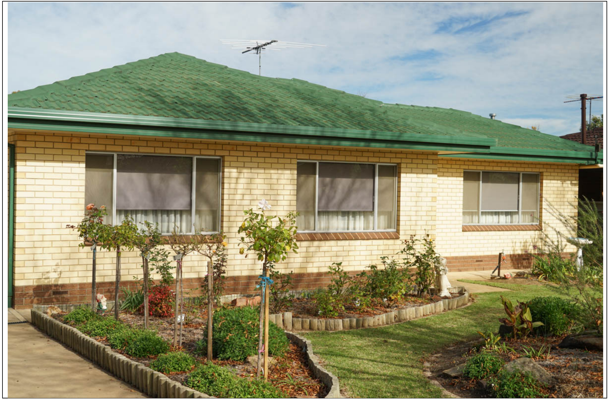
Photograph showing the exterior wall of the property, having no form of damage that could be related to tree root action.
