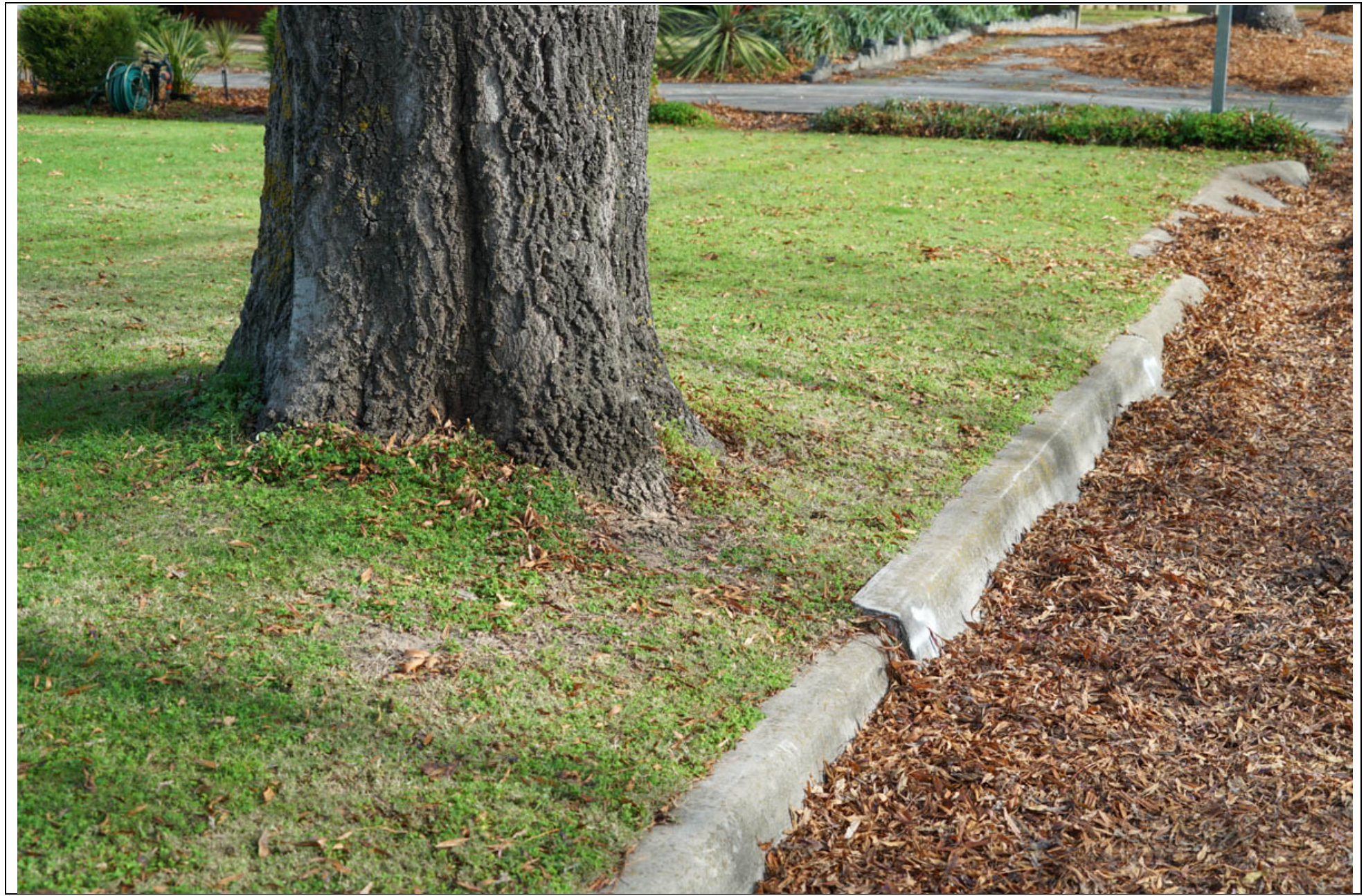
Photograph showing the minor kerb displacement adjacent to the stem of the tree.
