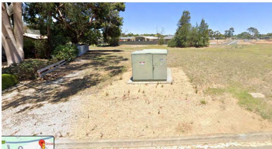
Figure 2 - street view Drinkwater Crescent, Nuriootpa - showing existing transformer.
